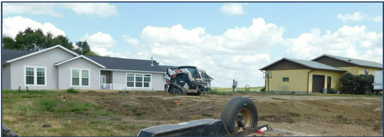
FIGURE 2 LOOKING NORTH FROM DRIVEWAY, BLUE HOME REMOVED (SITE OF PROPOSED NEW MOBILE HOME)
